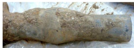
Exhibit 5-5: Lead Pipe at a Curb Stop
